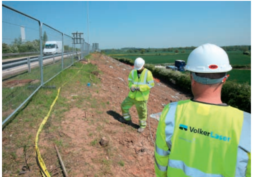
Access to site was gained from a field adjacent to the road and the carriageway remained open
