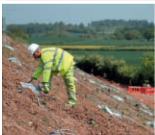
Pg 21 Charging the earth
